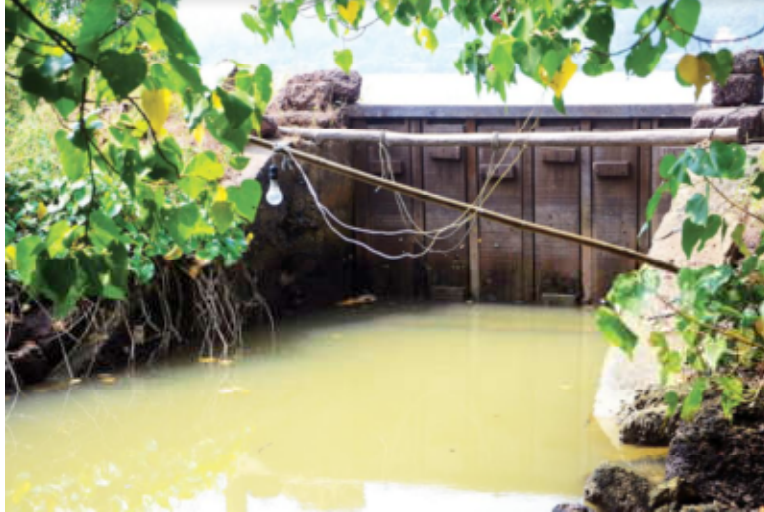
Three tier embankments: flap doors that help to regulate water movement to protect khazan lands
